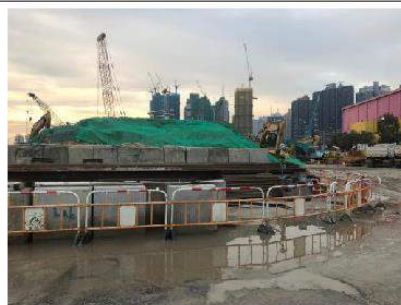
Covering stockpile of dusty materials completely when no work is being conducted
